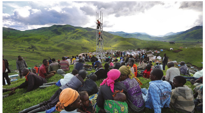
2 Villagers gather to watch the event as workers build the 18-meter tower.
